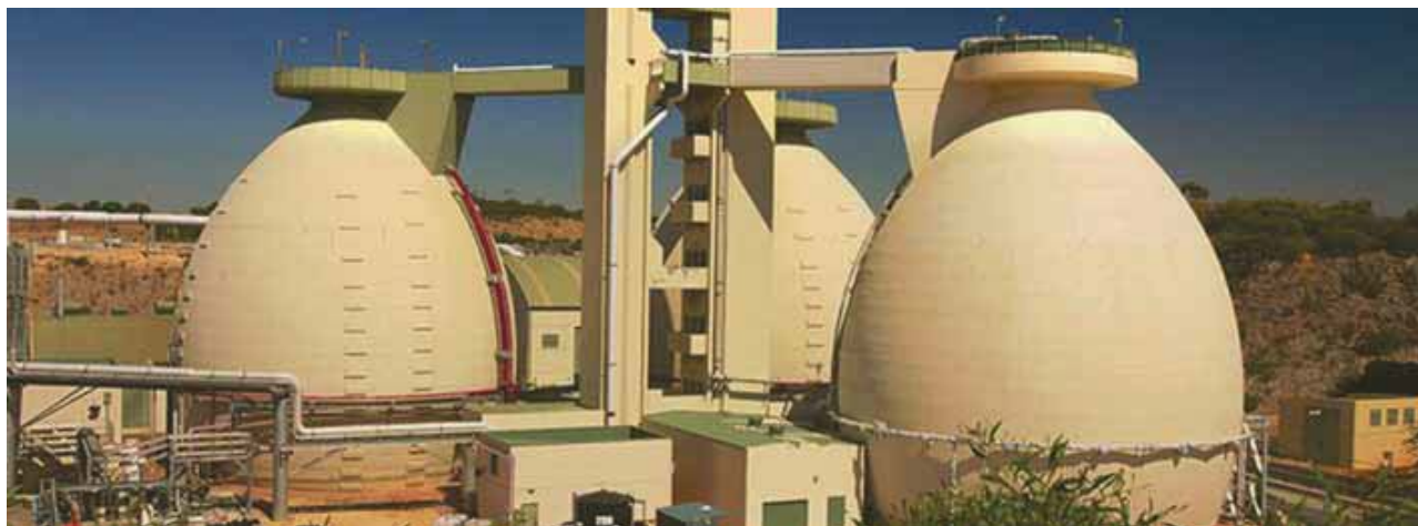
Figure 2. Egg-shaped digesters at Woodman Point WWTP. At 38 metres high, they are the largest of their type in the Southern Hemisphere.
